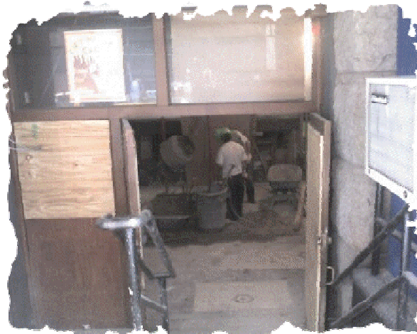
Construction is already underway at the future home of Kiddie Korner at the corner of Montague & Clinton Streets
